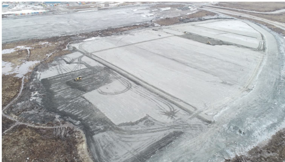
Figure 20-30 – An Aerial View of Filtered Tailings
